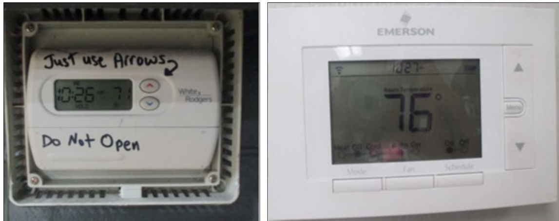
FIGURE 32: TYPICAL THERMOSTATS – SITE 2 (LEFT) AND SITE 4 (RIGHT). NO ALARMS DISPLAYED DESPITE ALARM CONDITIONS.
