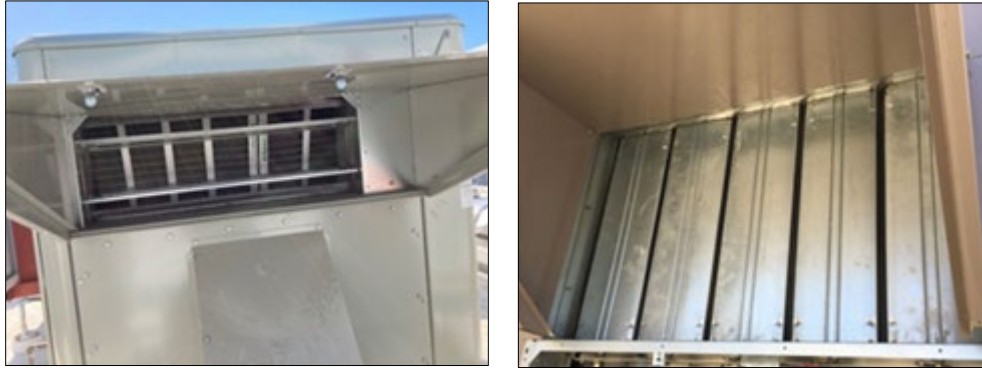
FIGURE 2: OUTSIDE AIR DAMPERS - 100% OPEN (LEFT) & FULLY CLOSED (RIGHT)
