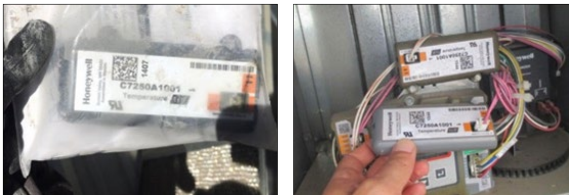
FIGURE 25: MIXED AIR SENSOR NOT INSTALLED – SITE 9 (LEFT) AND SITE 4 (RIGHT)
