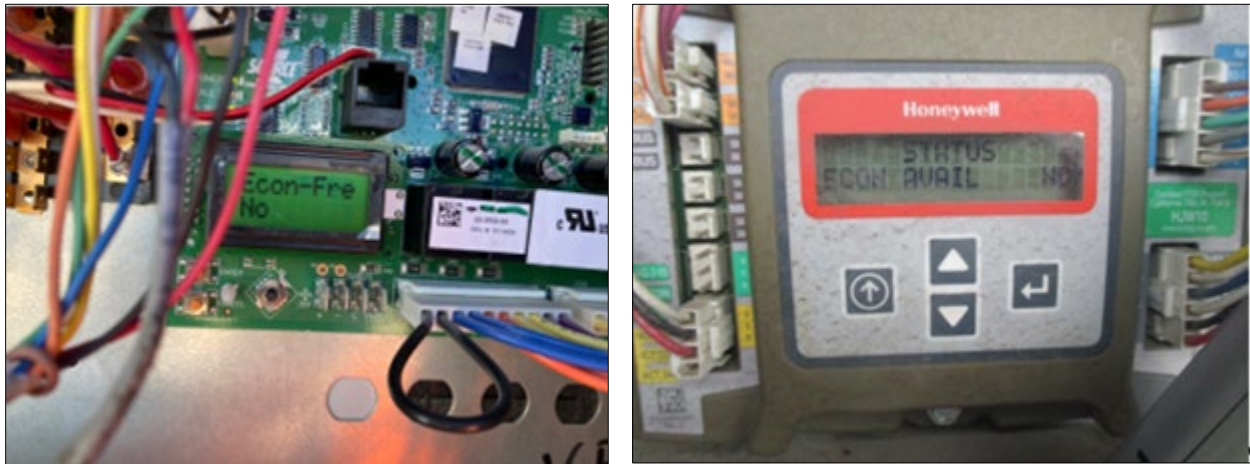
FIGURE 29: ECO (LEFT) AND JADE (RIGHT) CONTROLLERS DISPLAYING ECONOMIZER STATUS. BOTH SHOW NO ECONOMIZING AVAILABLE DUE TO OUTSIDE AIR TEMPERATURE ABOVE THEIR RESPECTIVE HIGH-LIMIT SETPOINTS.
