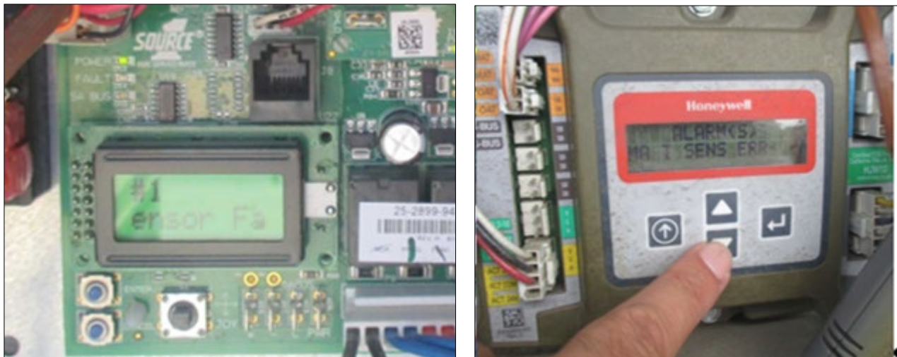
FIGURE 30: ECO (LEFT) AND JADE (RIGHT) CONTROLLERS. BOTH DISPLAYING SENSOR ERROR ALARM FAULTS AS MIXED AIR SENSORS WERE NOT INSTALLED
