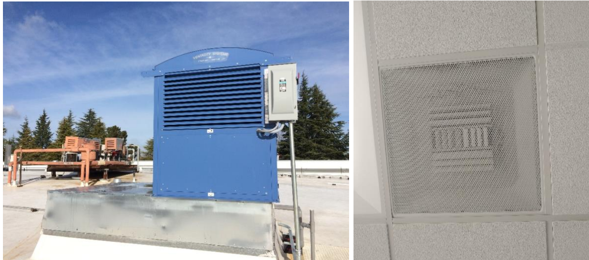
FIGURE 1: LEFT: NEW HRV-DOAS UNIT (FOREGROUND, RIGHT) AND EXISTING NATURAL GAS HEATING HOT WATER BOILER (BACKGROUND, LEFT); RIGHT: HRV-DOAS VENTILATION SUPPLY AIR DIFFUSER
