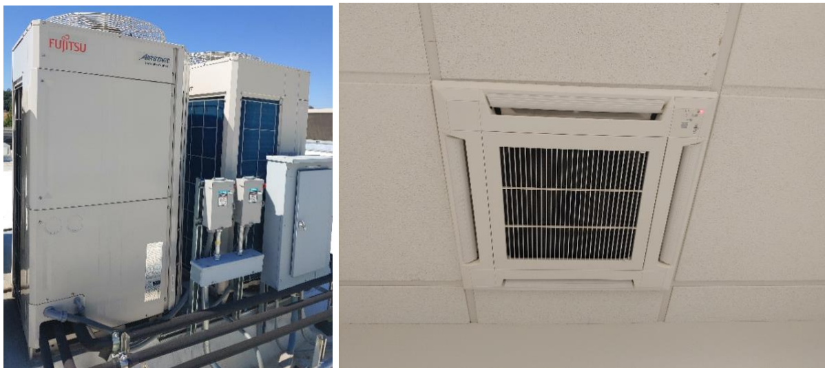
FIGURE 2: LEFT: NEW VRF OUTDOOR HEAT PUMPS; RIGHT: NEW VRF INDOOR FAN COIL CASSETTE
