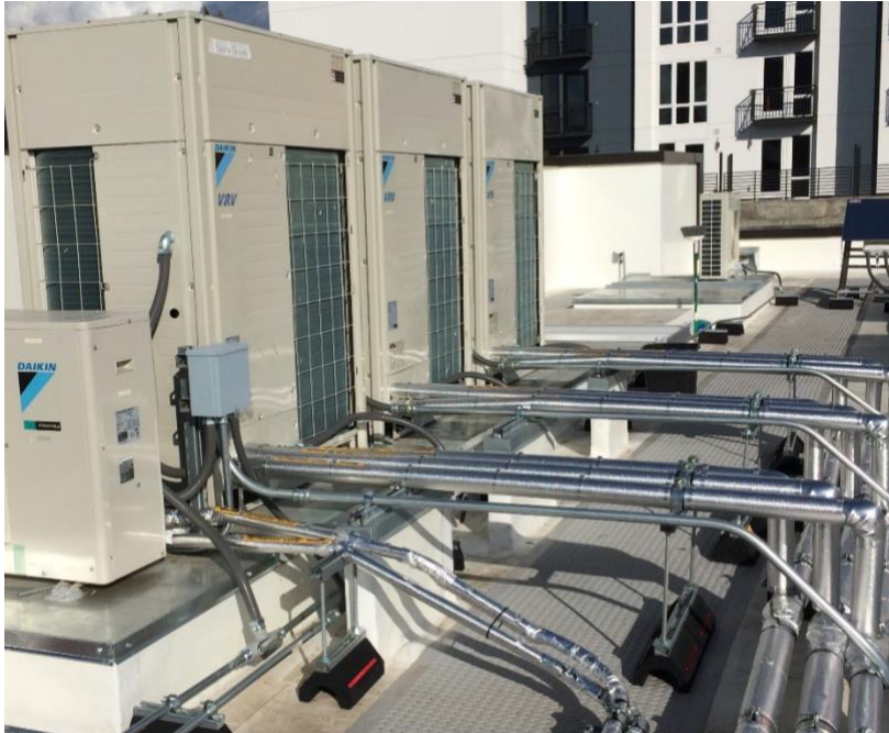
FIGURE 2: NEW VRF OUTDOOR HEAT PUMP (3 MODULES)
