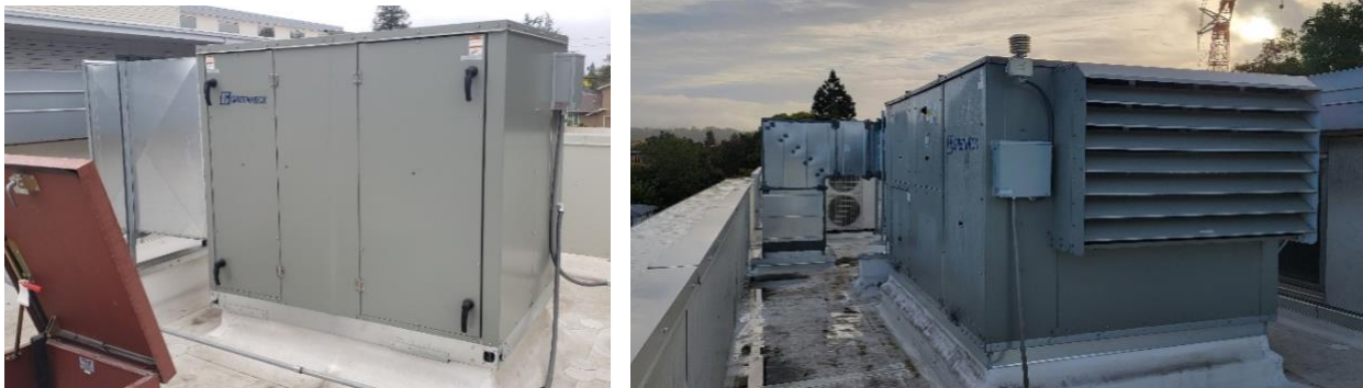
FIGURE 5: BUILDING B ERV-DOAS UNIT (LEFT) AND BUILDING A ERV-DOAS UNIT (RIGHT)
