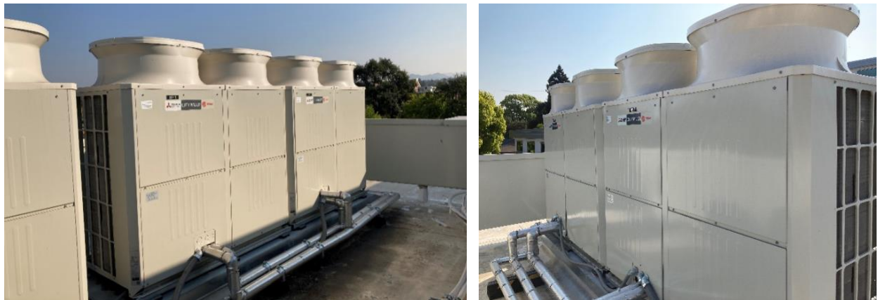
FIGURE 6: VRF OUTDOOR HEAT PUMPS, BUILDING A (LEFT), BUILDING B (RIGHT)
