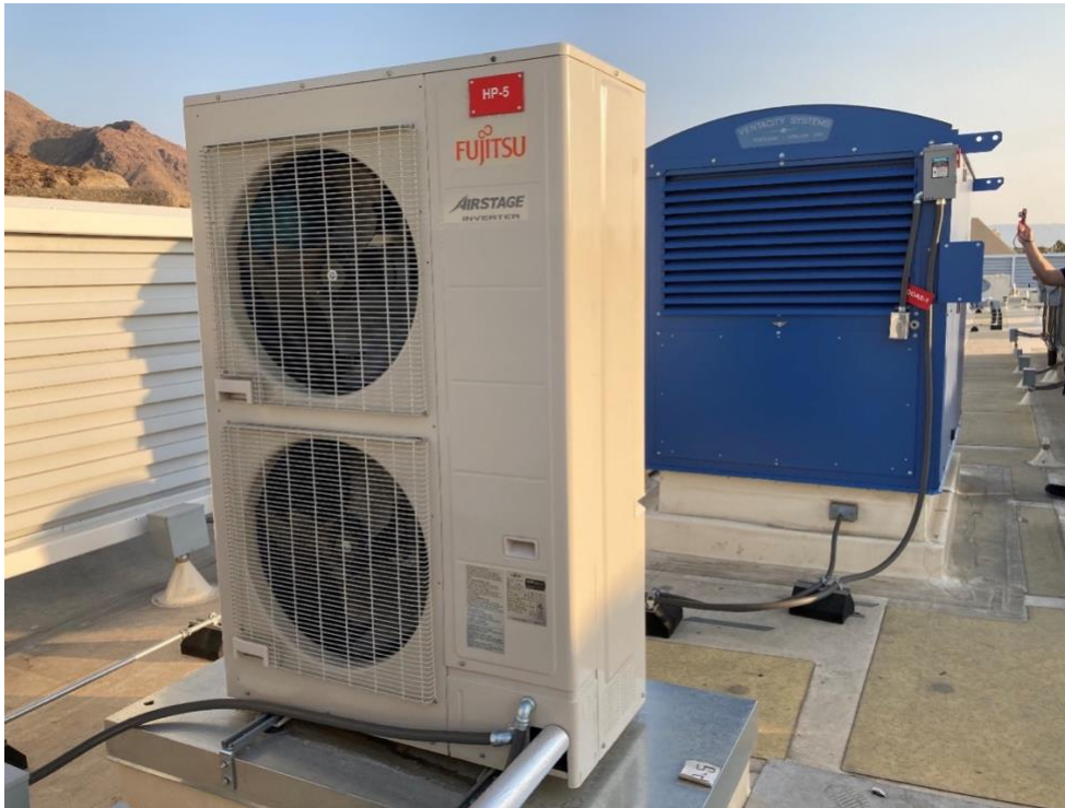
FIGURE 2: ERV-DOAS UNIT (BACKGROUND, RIGHT) AND ASSOCIATED HEATING & COOLING HEAT PUMP (FOREGROUND, LEFT)
