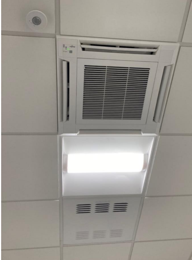
FIGURE 4: VRF CASSETTE FAN COIL (UPPER) AND DOAS SUPPLY AIR DIFFUSER (LOWER)
