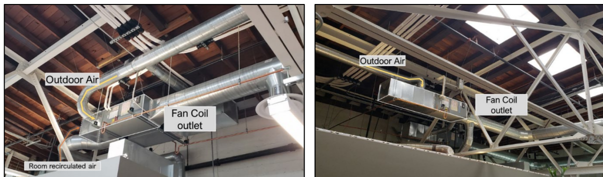
FIGURE 37: SITE PHOTO OF OAKLAND HVAC DISTRIBUTION DUCTING
