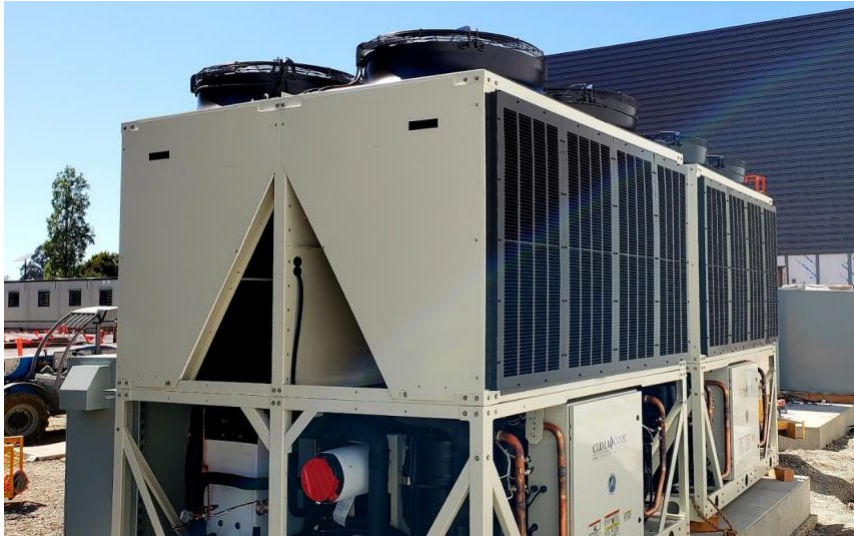
FIGURE 7: AIR-TO-WATER HEAT PUMP PHOTO
